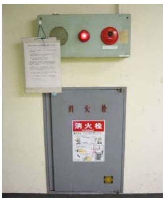
Fig.4. Fire alarm (top) and fire hydrant (below)
