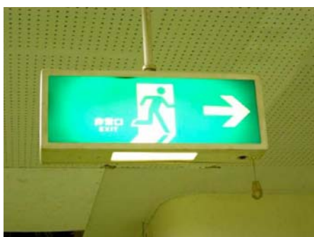
Fig.2. Lights indicating evacuation routes
