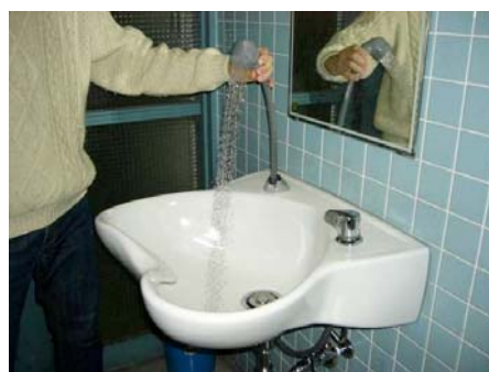
Fig.3. Emergency showers (located in washrooms)
