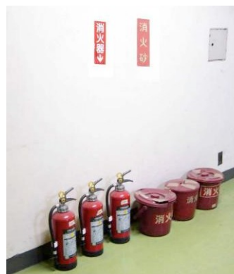
Fig.5. Fire extinguishers and fire extinguishing sand
