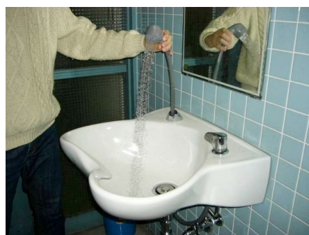
Fig.3. Emergency showers (located in washrooms)
