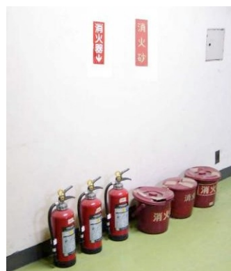
Fig.5. Fire extinguishers and fire extinguishing sand
