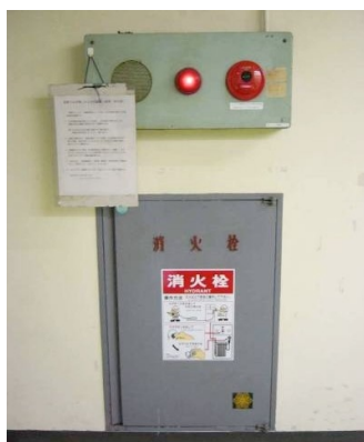
Fig.4. Fire alarm (top) and fire hydrant (below)
