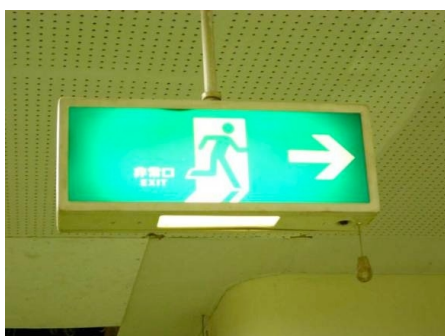
Fig.2. Lights indicating evacuation routes
